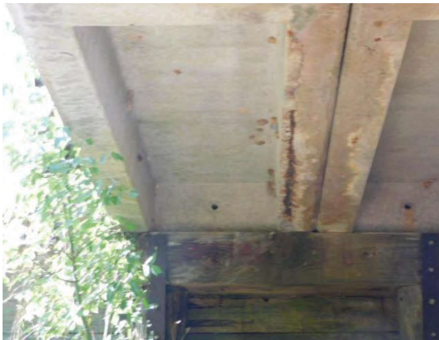
SLAB F SPAN 1 SPALLED TO STEEL
