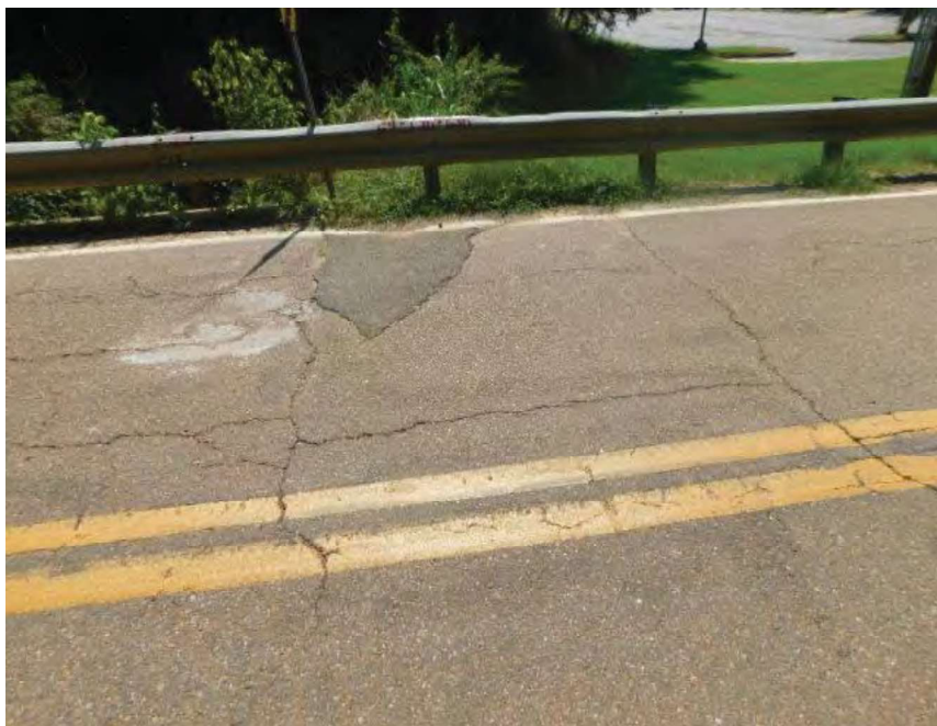
APPROACH 1 PATCHED, SETTLED
